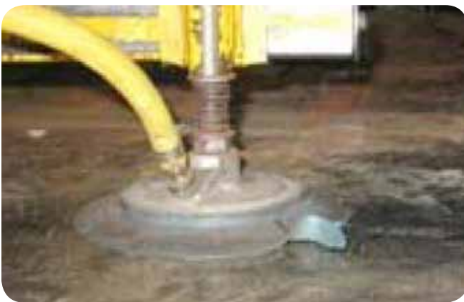
One of the many improvements of the 5S process involve equipment maintenance. Here, a jib crane lift cup shows signs of damage and is flagged for replacement.
